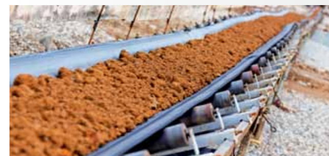
Part of the ore transportation system
