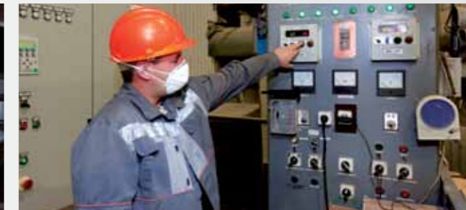
Checking plant control equipment
